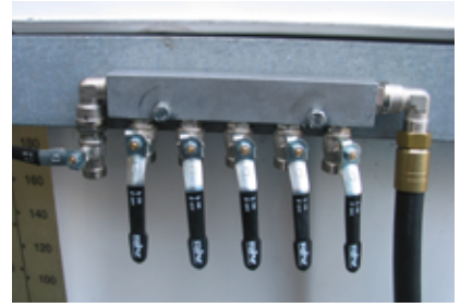
Collector at 6 cocks valve to operate with 6 users at same time
