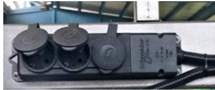
③ EXTERNAL ELECTRICAL OUTLET
